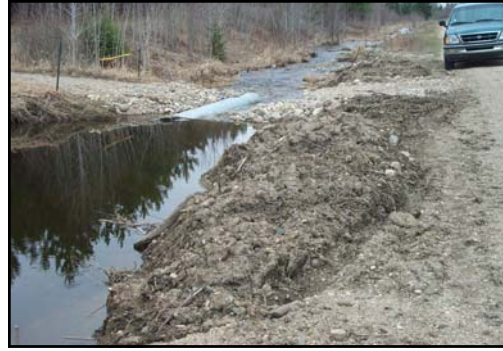
Channelized portion Before Project: Severe erosion, sedimentation and encroachment on township road. 2001 photo
