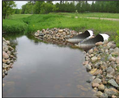
Completed Project (Downstream Crossing): New culverts, Rock Rip-Rap Armoring, and vegetated streambank slopes. 2007 photo
