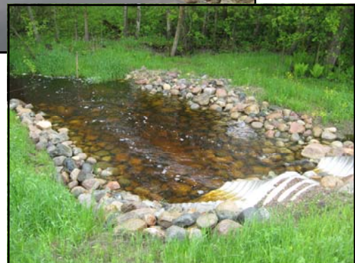
Completed Project (Downstream & Upstream Crossings): New culverts, Rock Rip-Rap Armoring, and vegetated streambank slopes. 2007 photo
