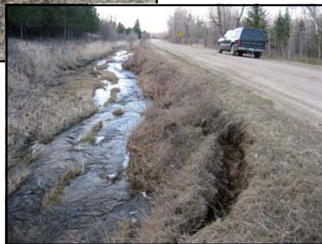
Channelized portion Before Project: Severe erosion, sedimentation and encroachment on township road.
